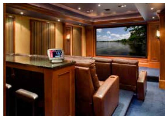
Custom Installation by Architectural Electronics, Inc., Winter Park, FL
